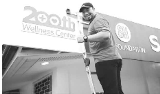
SM Foundation's Senior Project Manager Albert Uy places the 200th Wellness Center marker as they complete the final stages of the renovation.
