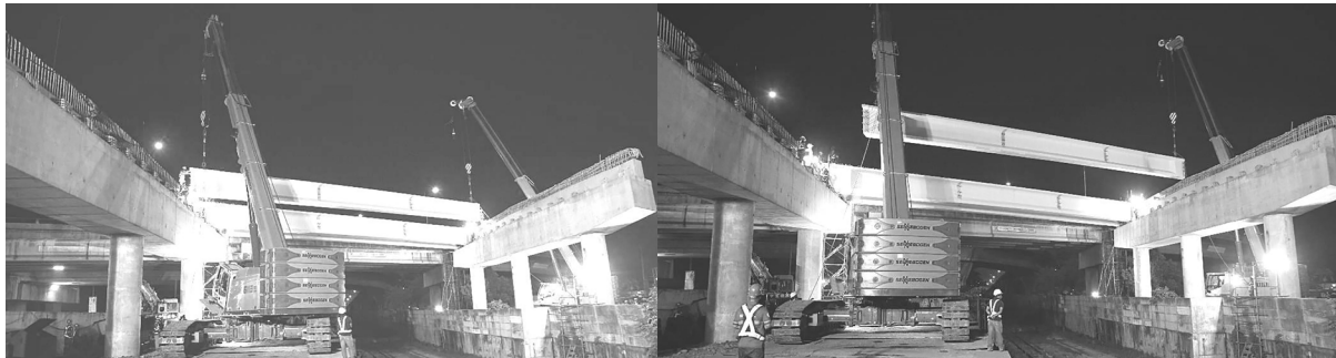
Actual photo of girder launching activity for CAVITEX C5 Link last 2018 over SLEX. Similar activity will be done at CAVITEX Paranaque (near Toll Plaza) for CAVITEX C5 Link R1 Interchange construction. During the girder launching activity starting September 15 to 24, 2023, counterflow lane will be activated for all vehicle classes.
