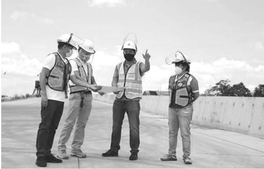
DPWH Secretary Mark A. Villar inspects CALAX Subsection 5 Santa Rosa, Laguna to Silang, Cavite. This 7.7km segment is targeted to open by third quarter of 2021. From L-r DPWH PPP Services Director Alex Bote, MPCALA VP for Tollways Development Engr. Art Monge, DPWH Sec. Mark A. Villar, BBB Committee Chair Ana Mae Lamentillo.
